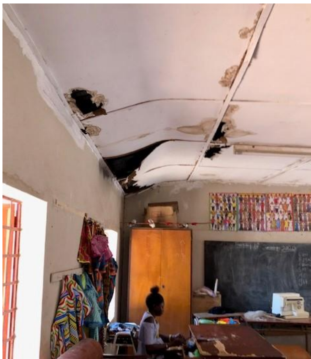
Ceiling damage, St. Peter's Skill Centre, Feb. 2020
